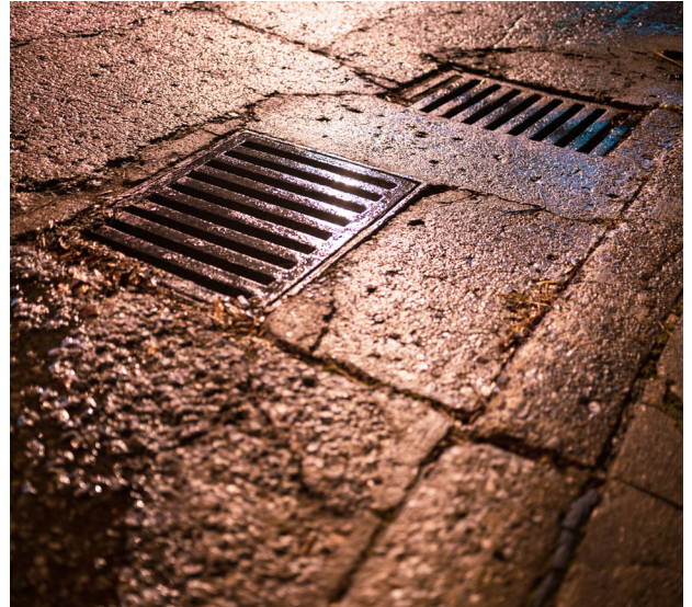
Data about underground drainage networks is scarce and costly to obtain. The CSHub is exploring the use of simulations to characterize flood risk with only surface data.
